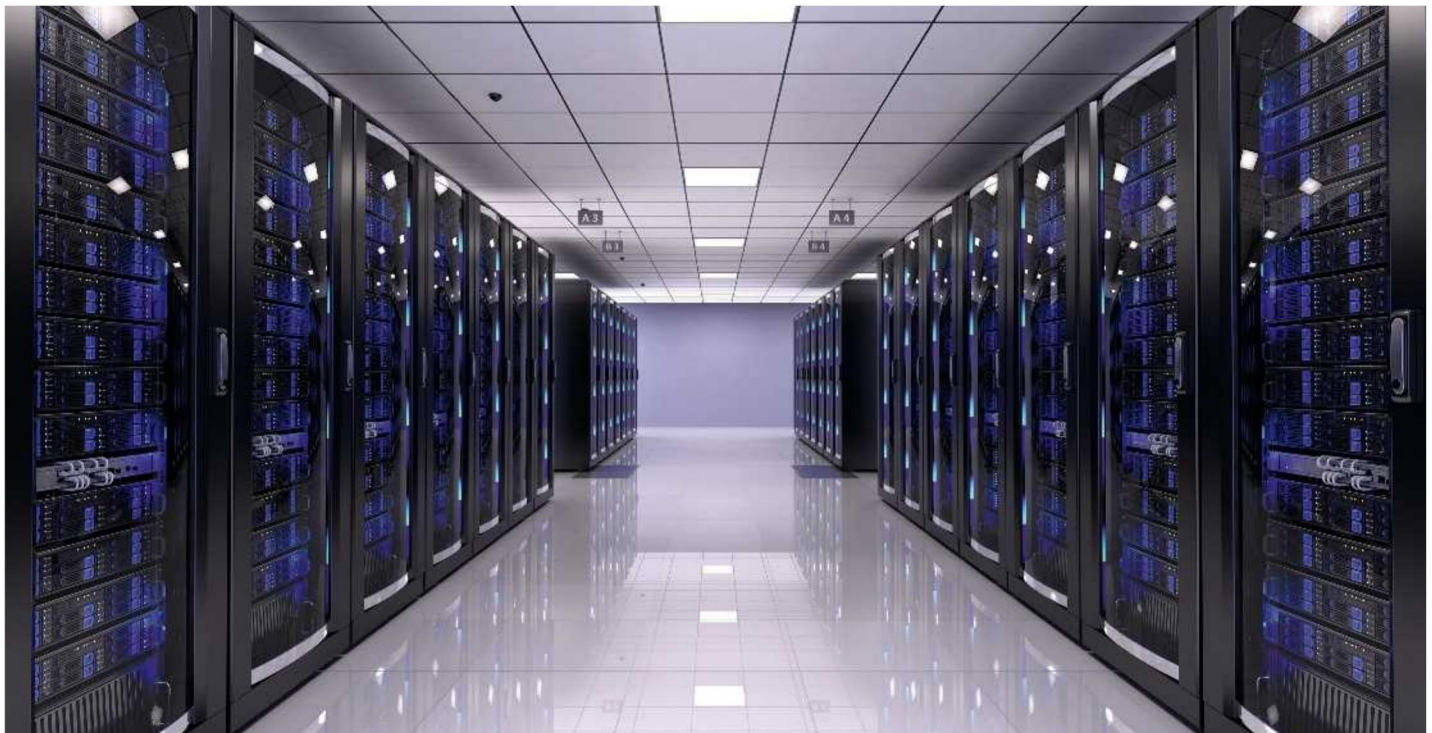
Fig. 68: Data center with a DC power supply system with linear source characteristics
